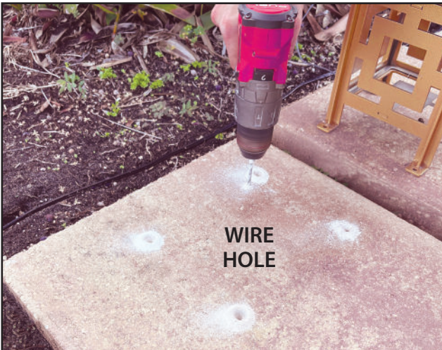
Drill 4 holes in the Deck for the feet attachment and one for landscape connection wire.
